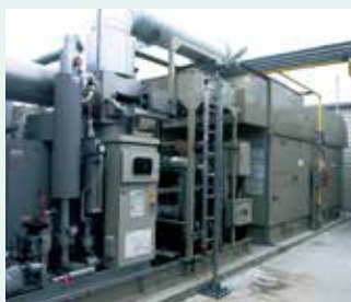
Co-generation system at Gifu Plant
