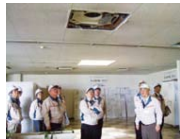
President Toyoda inspects damage at Toyota Boshoku Tohoku Corporation.
